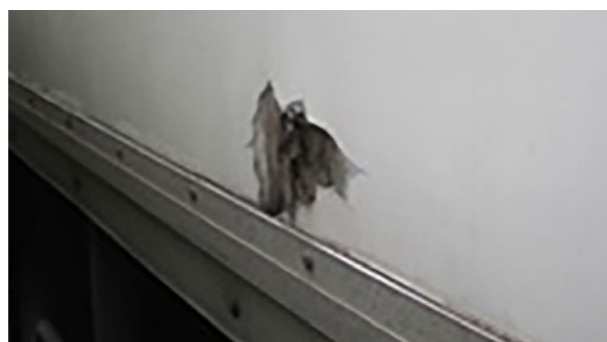
Wood side panels: Damaged wood support \geq 20\text{ cm}
